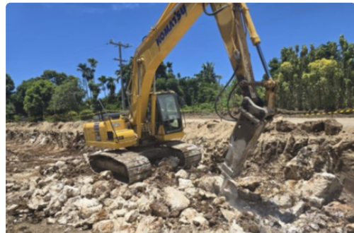
Upgrading and sealing of 2.5km from Chabbai Junction on Buka Road, Bougainville
